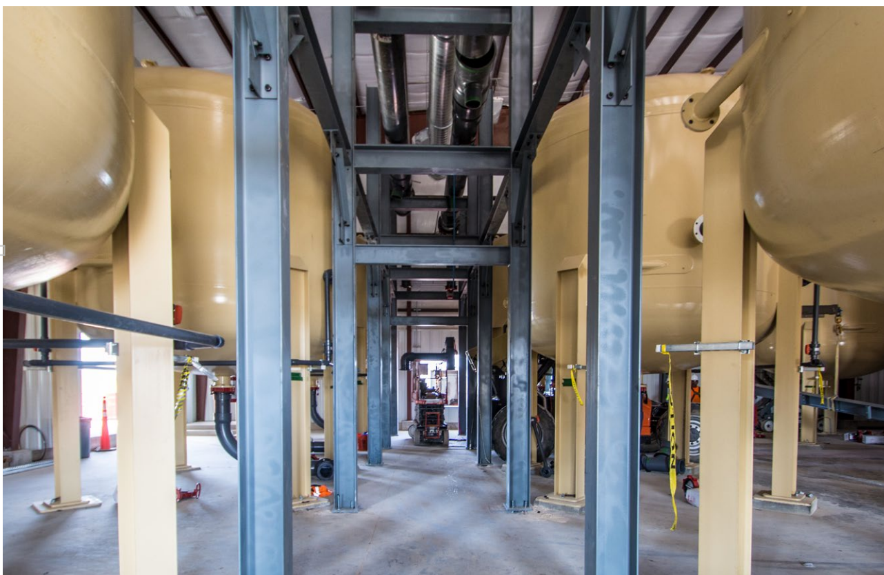
Figure 4: Completed Ion Exchange Columns within the CPP, Wyoming USA
