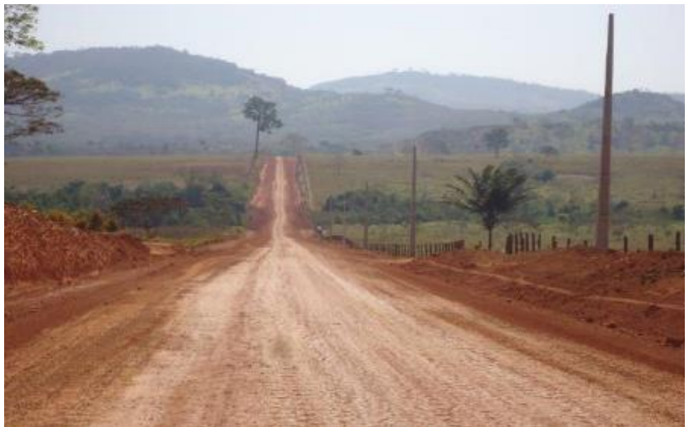
The mine access road, including construction of a number of river bridges, is ongoing
