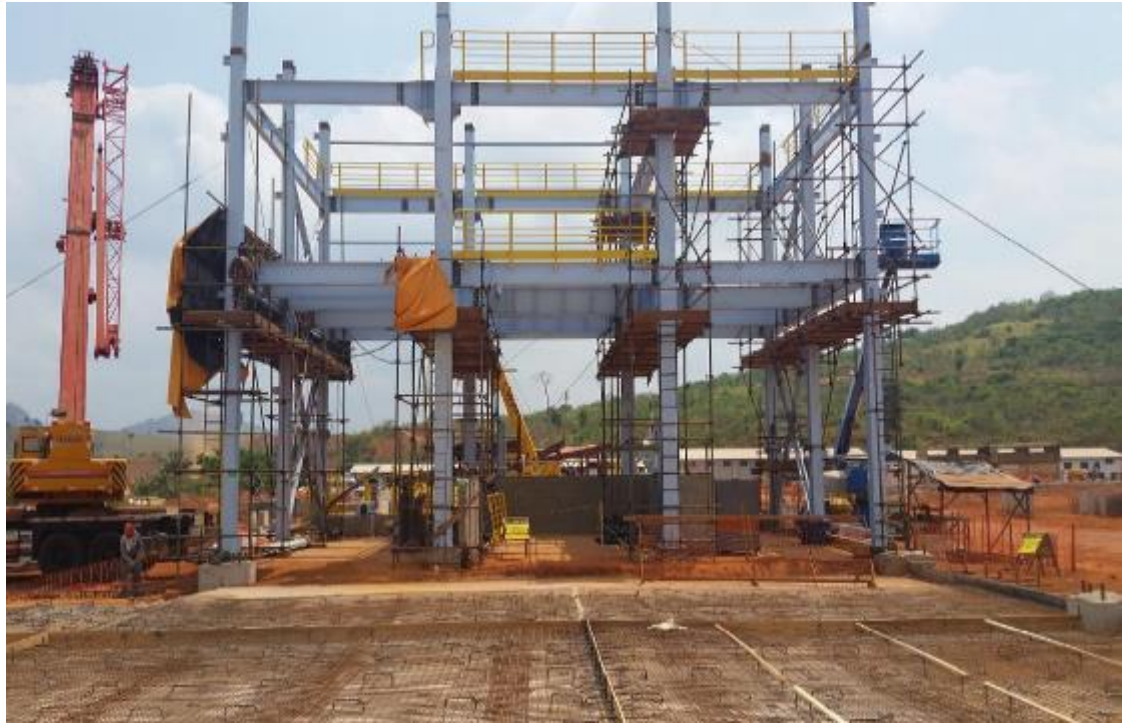
Filter House building footings are completed and structural steel building is progressing on schedule
