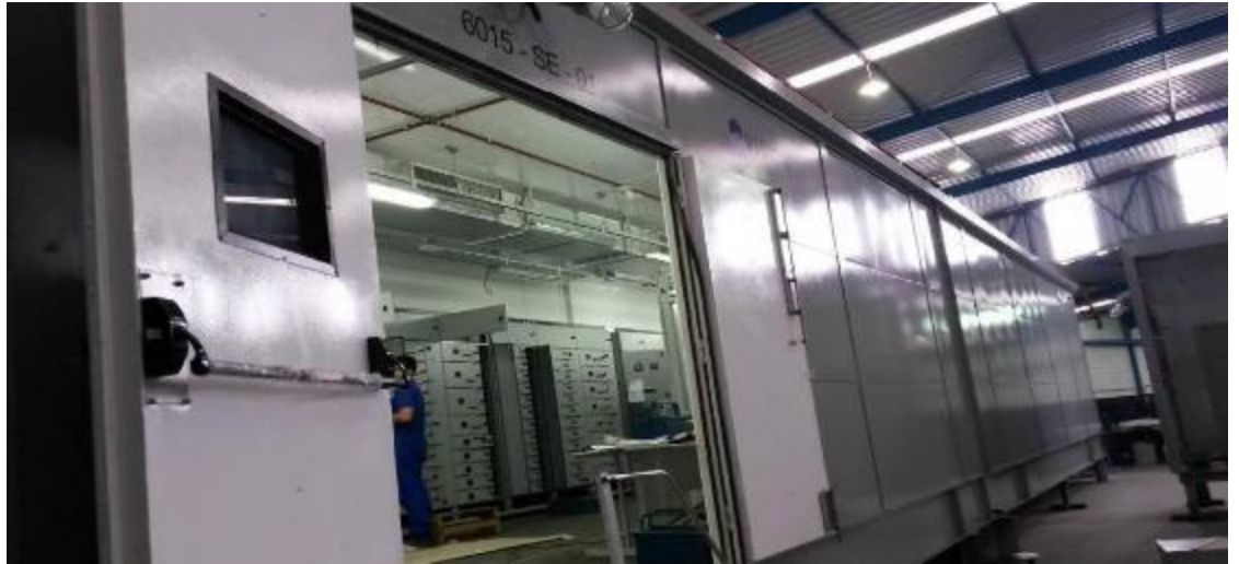
Flotation area electrical installation is simplified by the use/delivery of pre-wired Motor Control Centers
