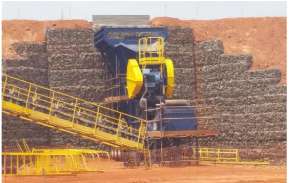
Earthworks associated with the initial ROM Pad construction are complete and the retaining wall erected. The jaw crusher is installed below the tip head, awaiting only the feed hopper, grizzly and electric
