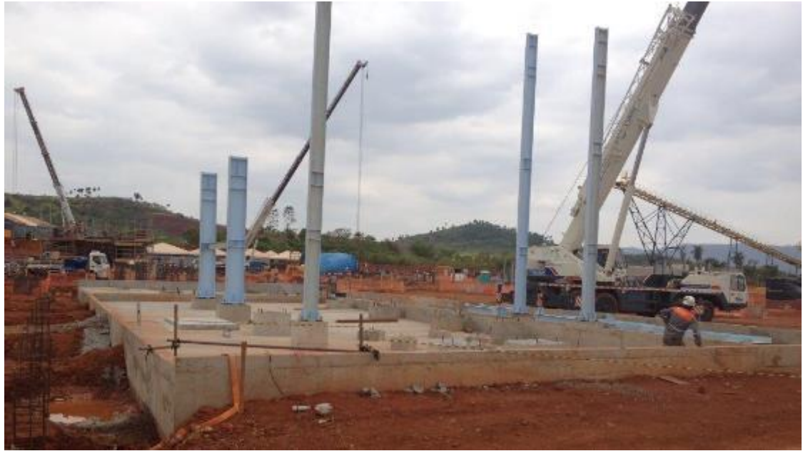
Flotation floor civils are sufficiently advanced to allow the start of structural steel to support the float cells
