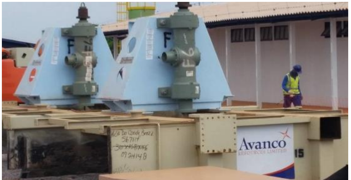
Rougher-Scavenger OK 38 Flotation Cells ready for lifting into position once the steel structures are ready
