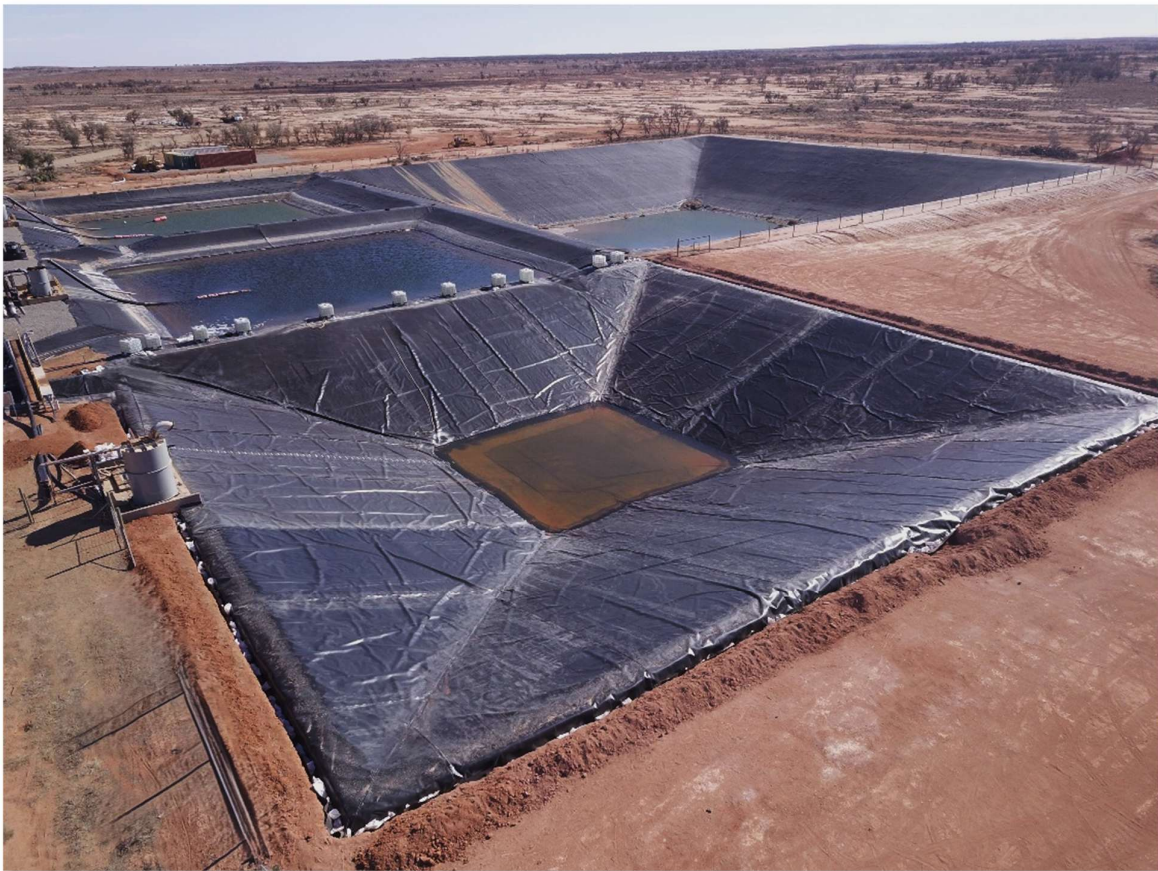
Figure 2; PLS (Pregnant Leach Solution) pond now approved for use at White Dam Gold Project, South Australia
