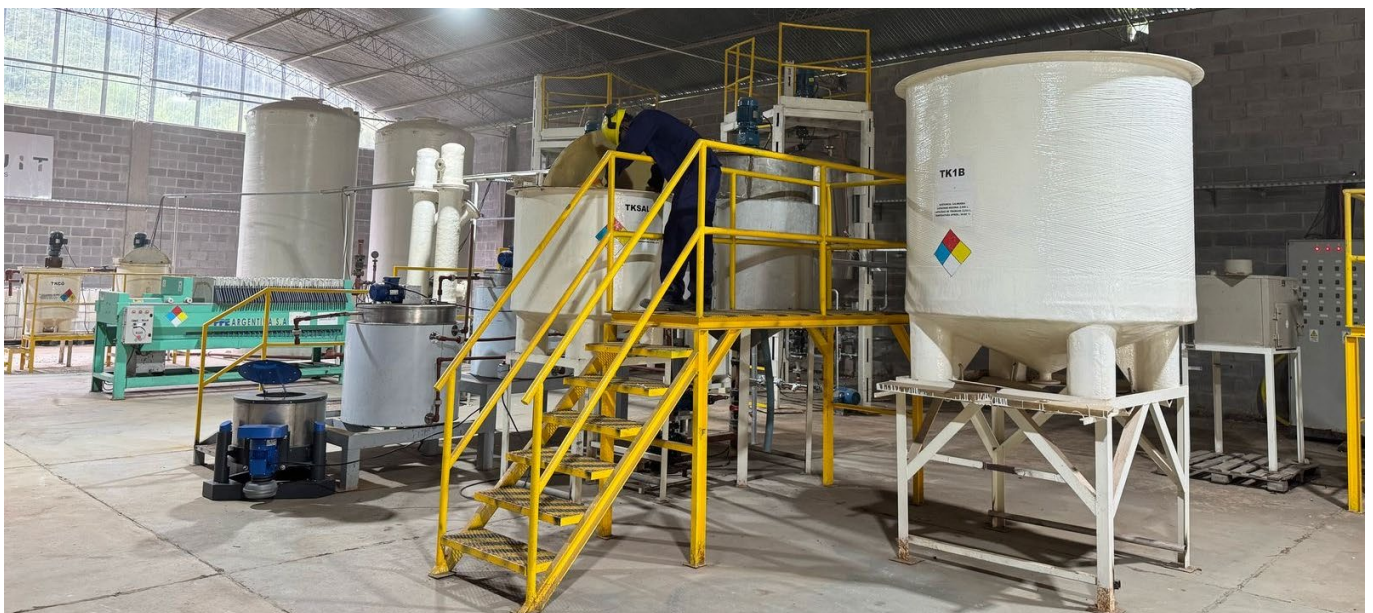
Figure 1 – Pursuit’s 250tpa Lithium Carbonate Pilot Plant in Salta, Argentina.
