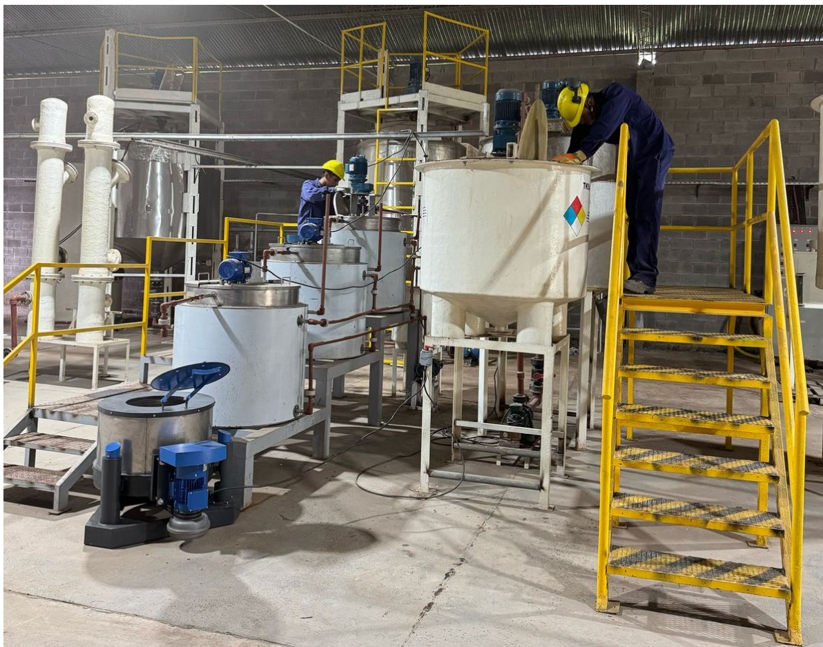
Figure 2 – Commissioning in Action: Pursuit Team Conducts Hydrostatic Testing at the Pilot Plant
