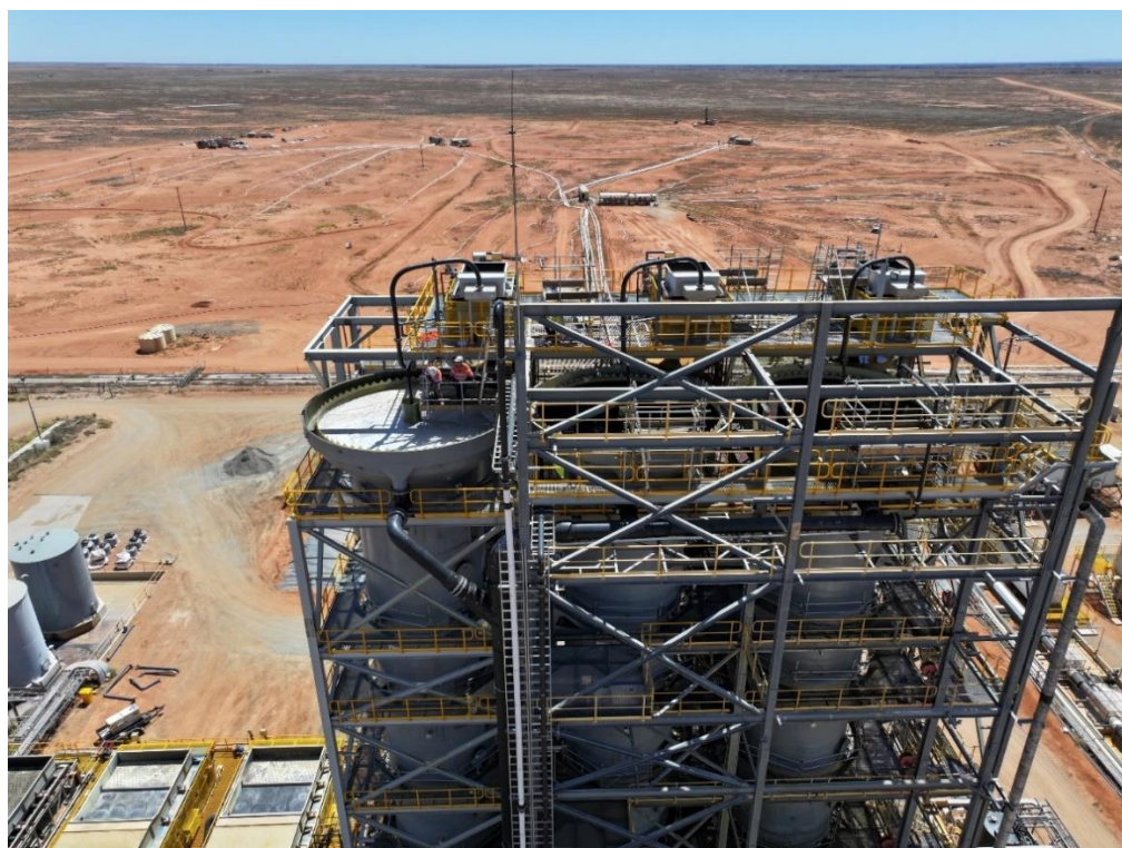
Figure 1: NIMCIX Column 3 Commissioned and in Operation
