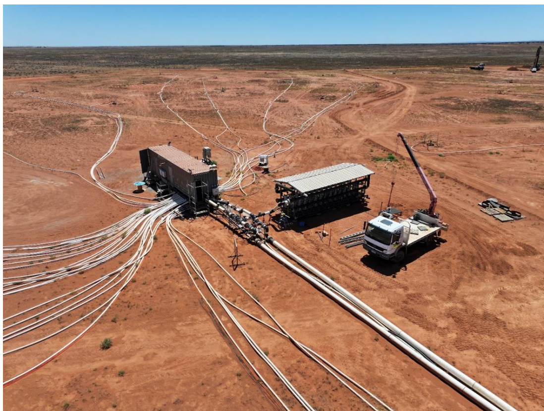
Figure 2: Wellfield 3 Flushed and Primed for Production
