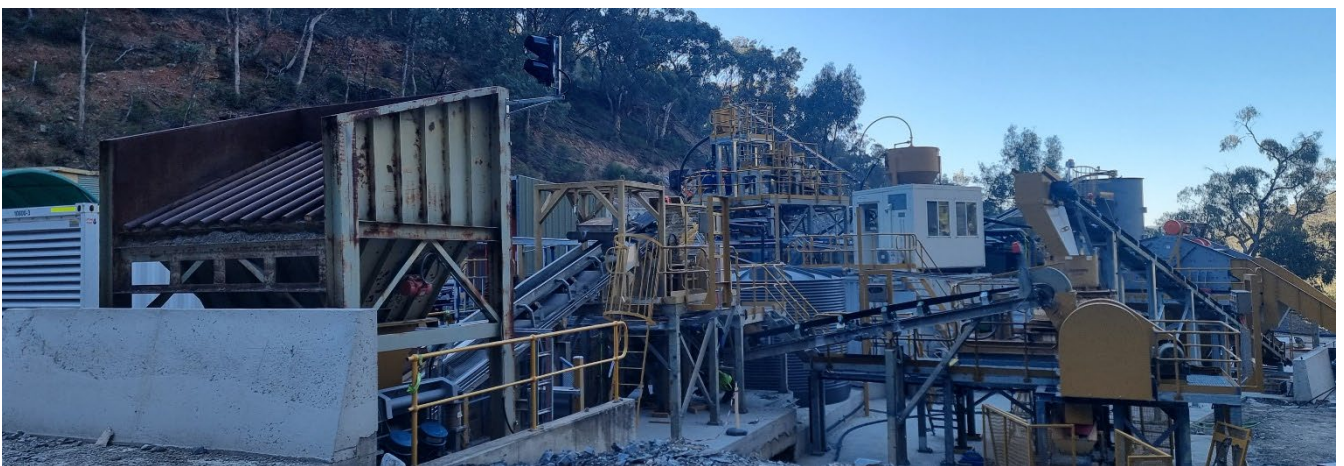
Figure 3 Reward gravity gold plant overview from the Feed hopper back over crushing circuit and gravity circuit
