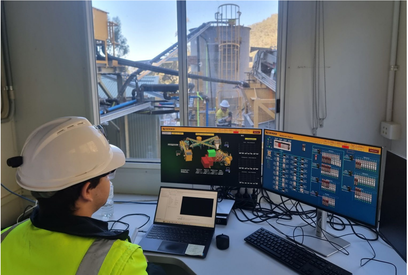
Figure 1 Automation programming technician testing the Reward gravity plants automations systems from the Control room
