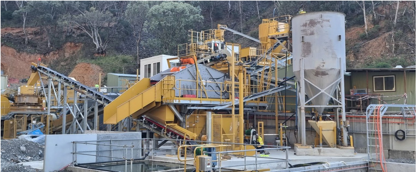
Figure 4 Reward gold gravity plant looking back over the crushing circuit
