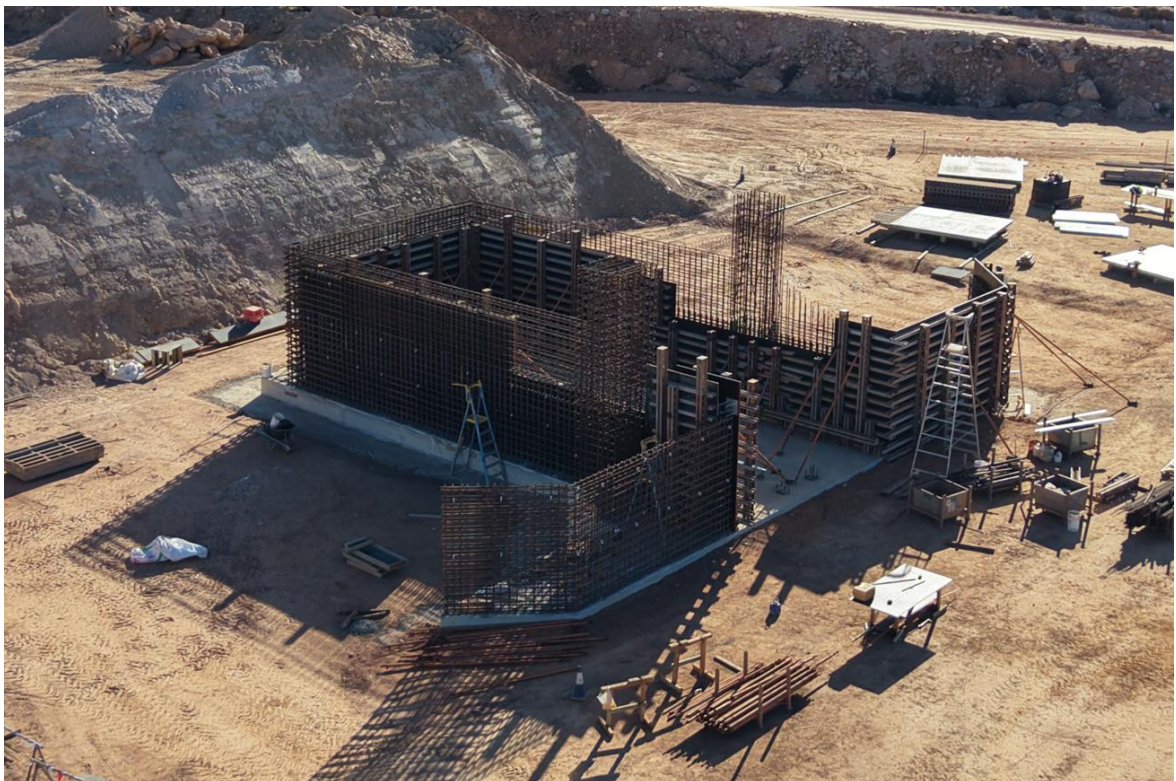
Figure 2 – Primary Crusher steelwork
