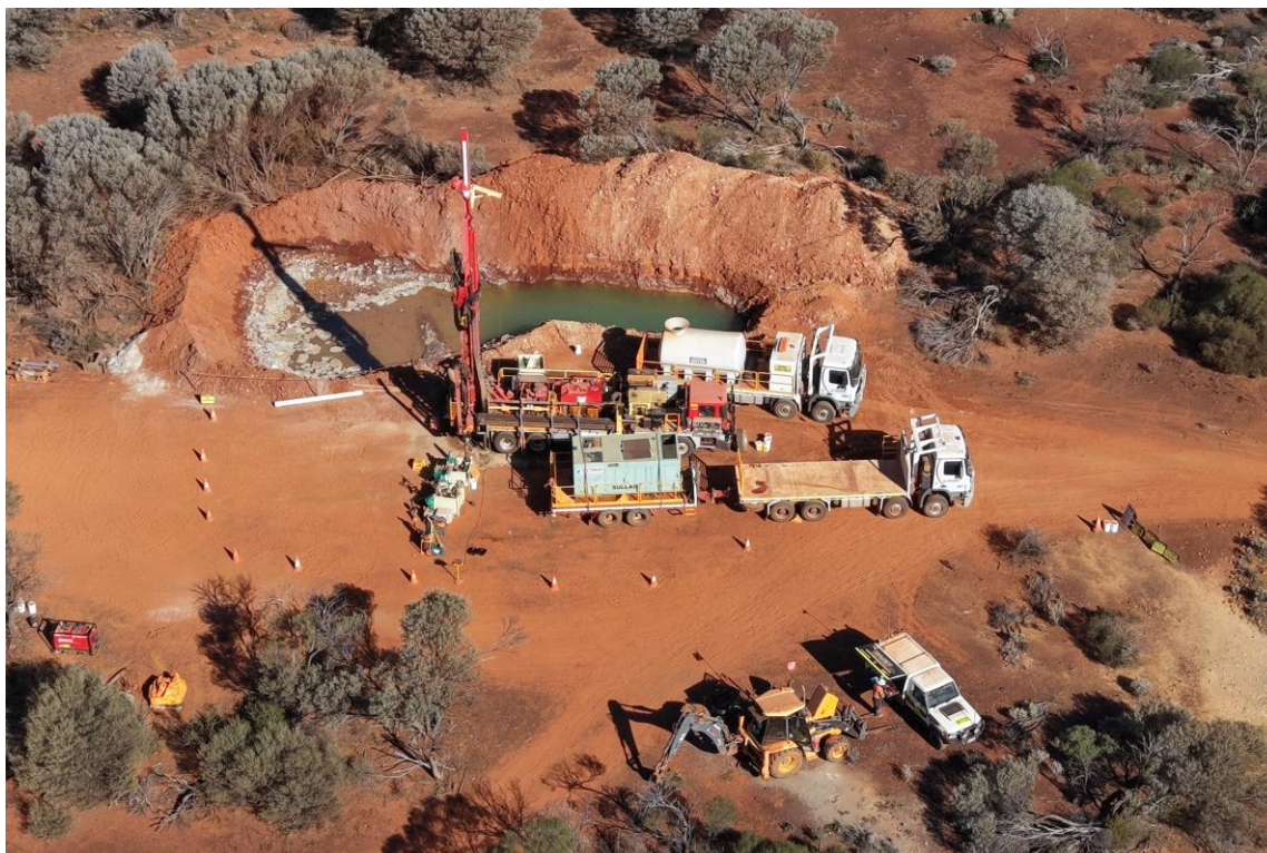
Figure 7 – Production borefields Development
