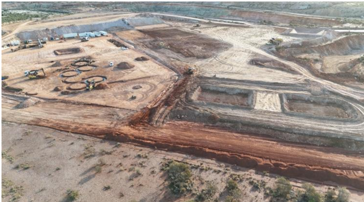
Figure 2 - Earthworks for the processing infrastructure (left) and the Process Water ponds (right) (28 June 2026)
