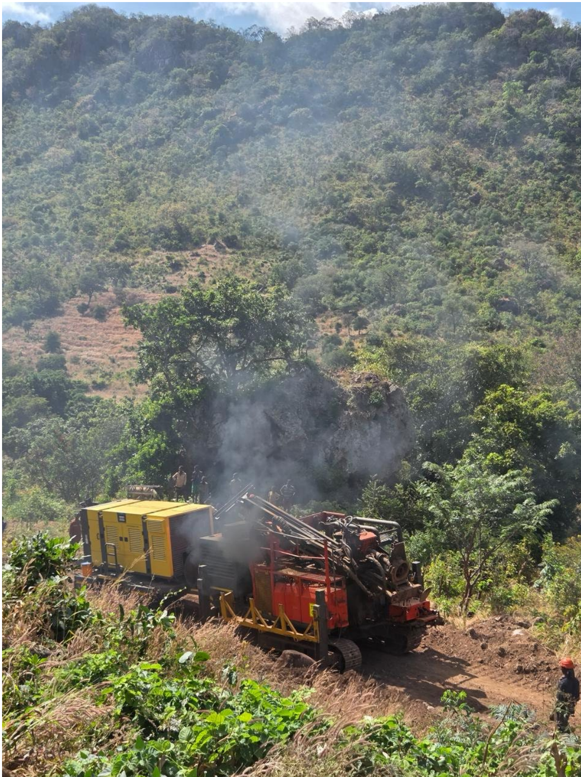
Figure 1 – Mobilising RC drill rig to drill pad for the first hole at Nathace Hill
